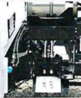
Secondary outside manual control valve with protective cover
